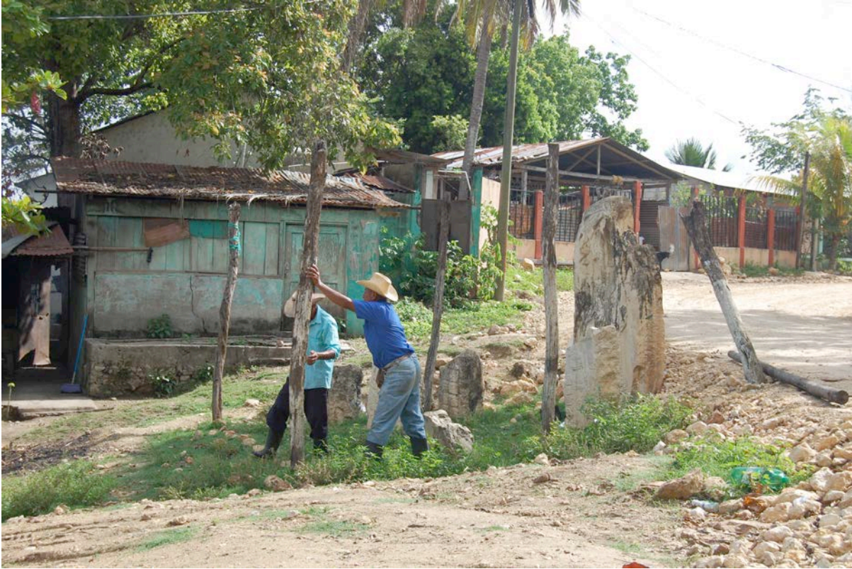
Rotten posts of old monument roof.
